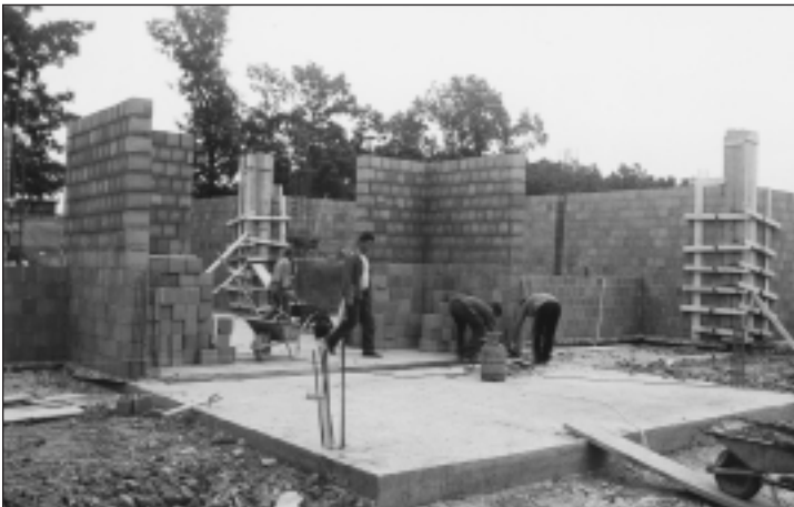
Emin Duraku school during an early stage of its construction by M-USA.
